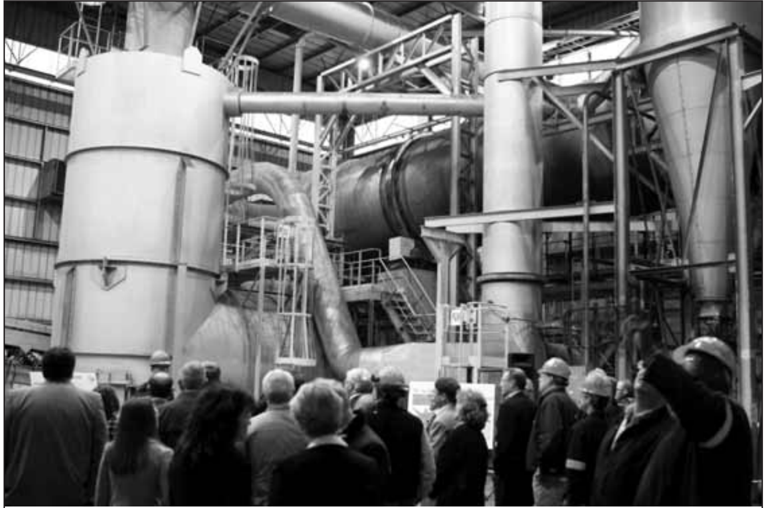
Guests of the event view new equipment installed as part of the expansion. The project includes a new crusher, furnace, state of the art environmental controls and associated handling equipment.
