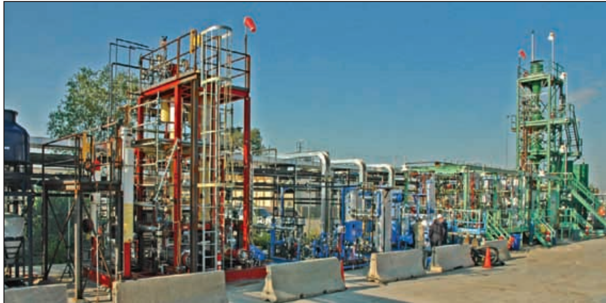
Range Fuels' plant located in Broomfield, Colorado will use wood waste to create ethanol.
