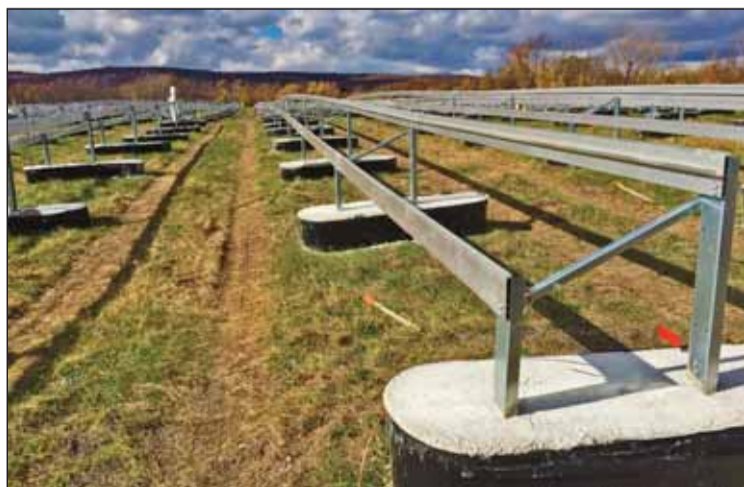
Concrete is poured in-place in plastic tubs to create ballasts to anchor solar racking and panels while minimizing the impact on landfill caps and speeding installation.
