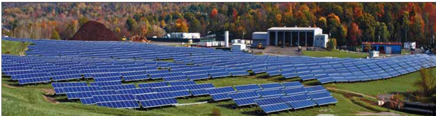
A two megawatt solar installation at a former town landfill in West Nyack, New York.
