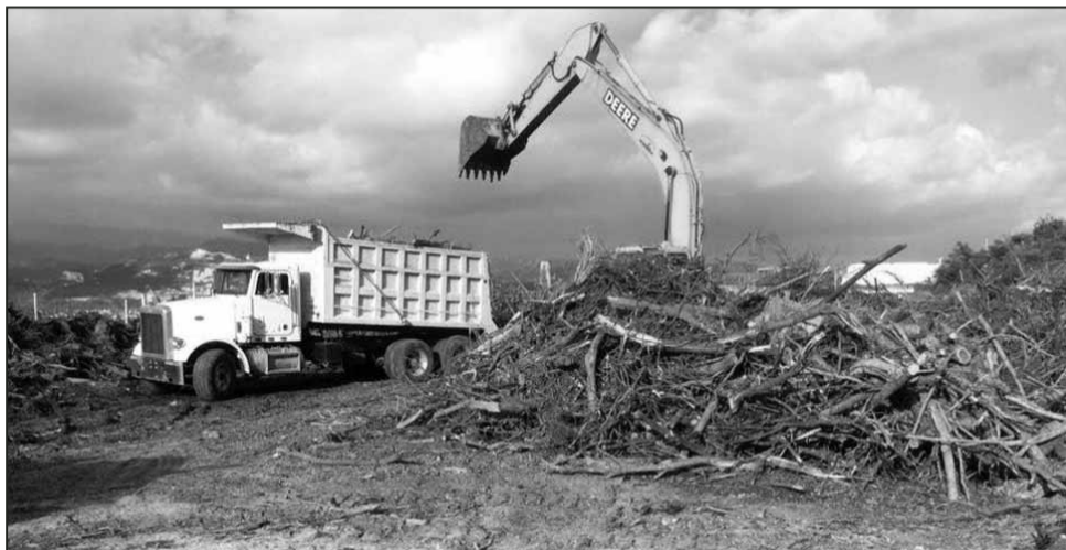
U.S. Army Corps of Engineers contractors remove Hurricane Maria debris from a temporary disposal site in Ponce, Puerto Rico. Approximately 630,000 cubic yards of vegetative debris will be reduced for composting and other uses. Construction and demolition debris such as lumber and household furniture is expected to yield about one million pounds of recyclable metals. PHOTO COURTESY OF U.S. ARMY
