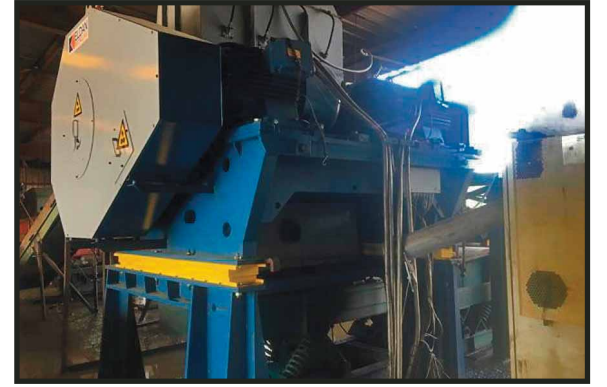
2014 ELKAN TIRE RASPER SYSTEM Includes magnets, baghouse and deluge system.
