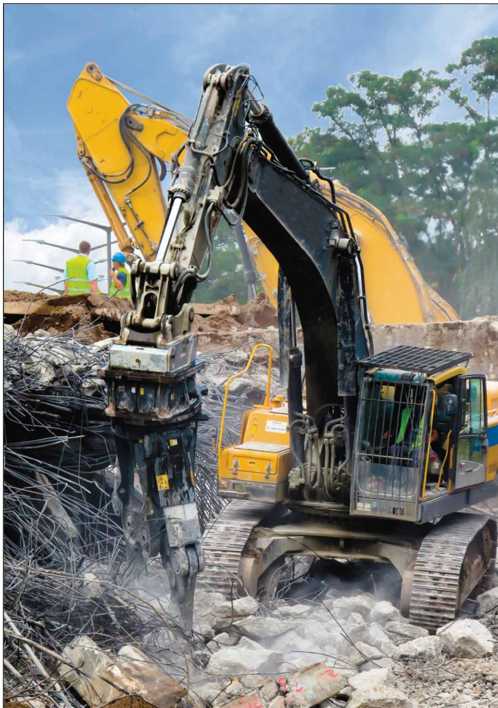
One of the current challenges to scrap metal recyclers is contamination when dealing with separating recyclable steel from various construction materials during building demolition. PHOTO BY GELLINGER | PIXABAY
