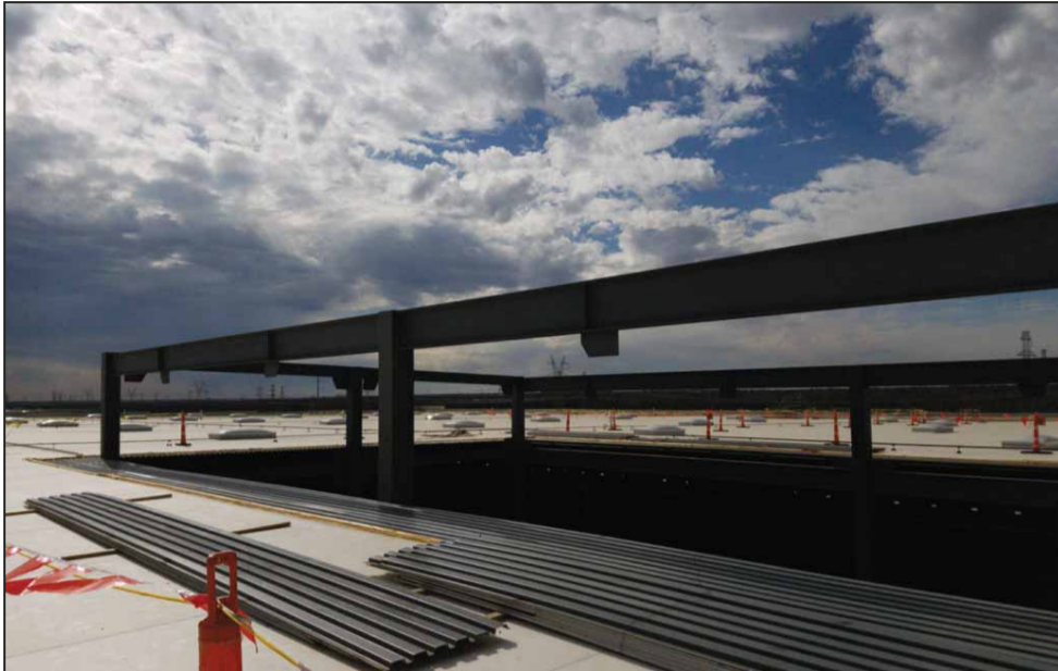
Plastic recycler CarbonLITE has engaged C1S Group as the primary contractor for the construction of a new North Texas recycling facility. C1S Group, a full-service professional engineering and construction firm based in Dallas, is converting an existing facility in southwest Dallas into a leading edge recycling center.
