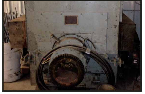
SIEMENS 1500 HP SHREDDER MOTOR 900 rpm, 3-phase, 4,000 volt.
