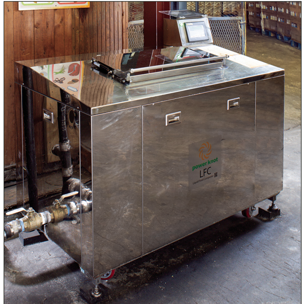
The LFC-200 biodigester in Jersey Lynne Farms' Brooklyn distribution warehouse is compact, quiet and odorless during continuous operation.
