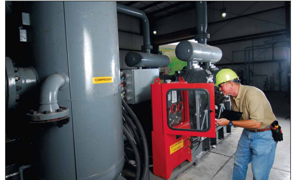
A look at the internal workings of one of Waste Management's many LFG projects.
