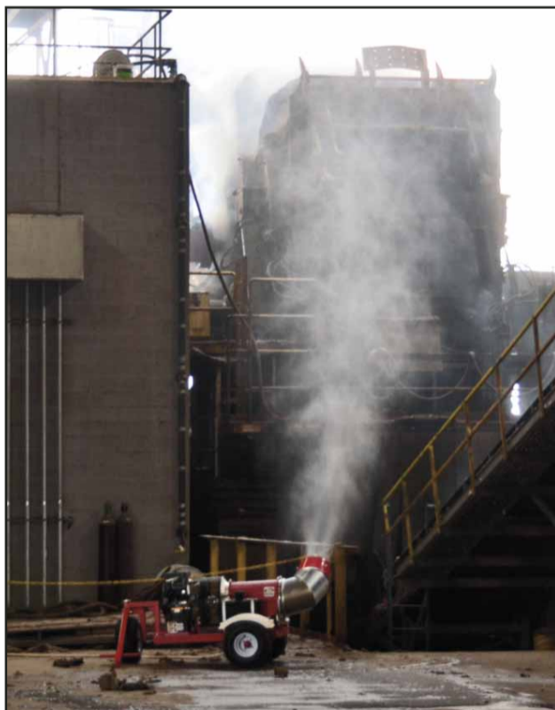
Buffalo Turbine LLC
