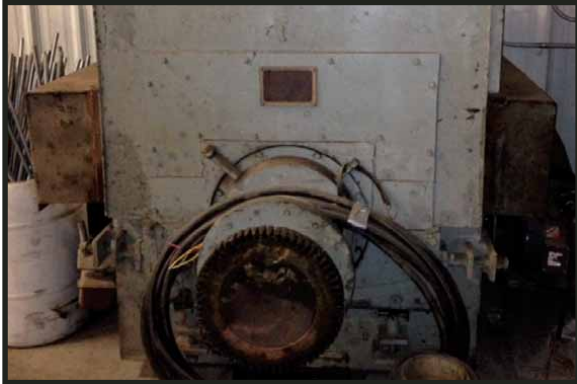
SIEMENS 1500 HP SHREDDER MOTOR 900 rpm, 3-phase, 4,000 volt.
