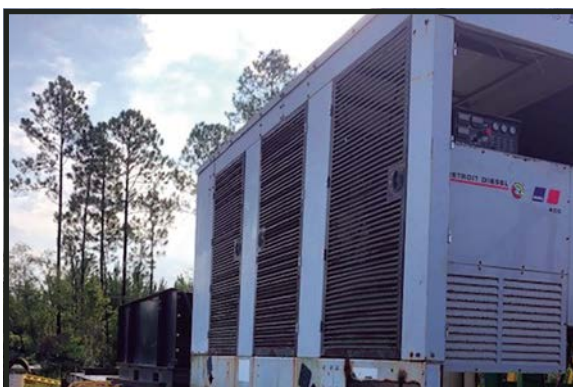
405KW DETROIT DIESEL GENERATOR
