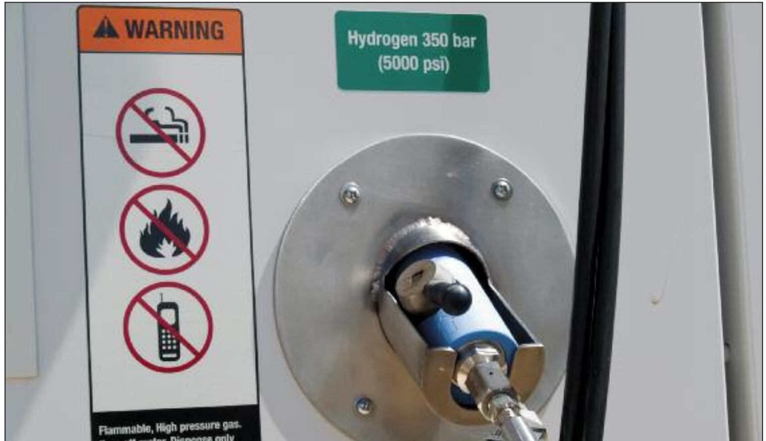
Close up of a hydrogen fueling dispenser for vehicles.
