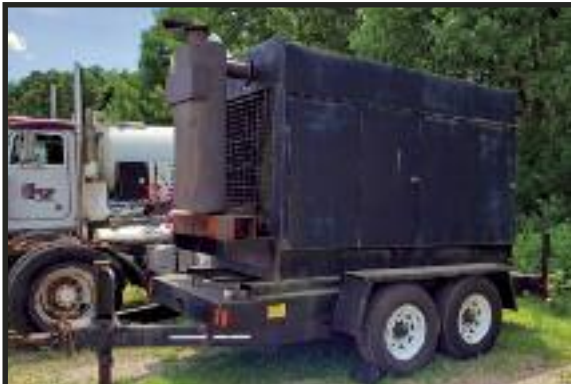
LEROY SOMER PORTABLE 250KW GENERATOR 60 Htz 3 phase 240/480 Volts John Deere Motor.
