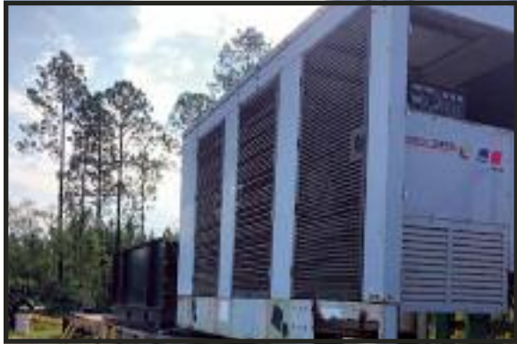
DETROIT DIESEL 425KW GENERATOR 240/480V three phase, 500 amps.
