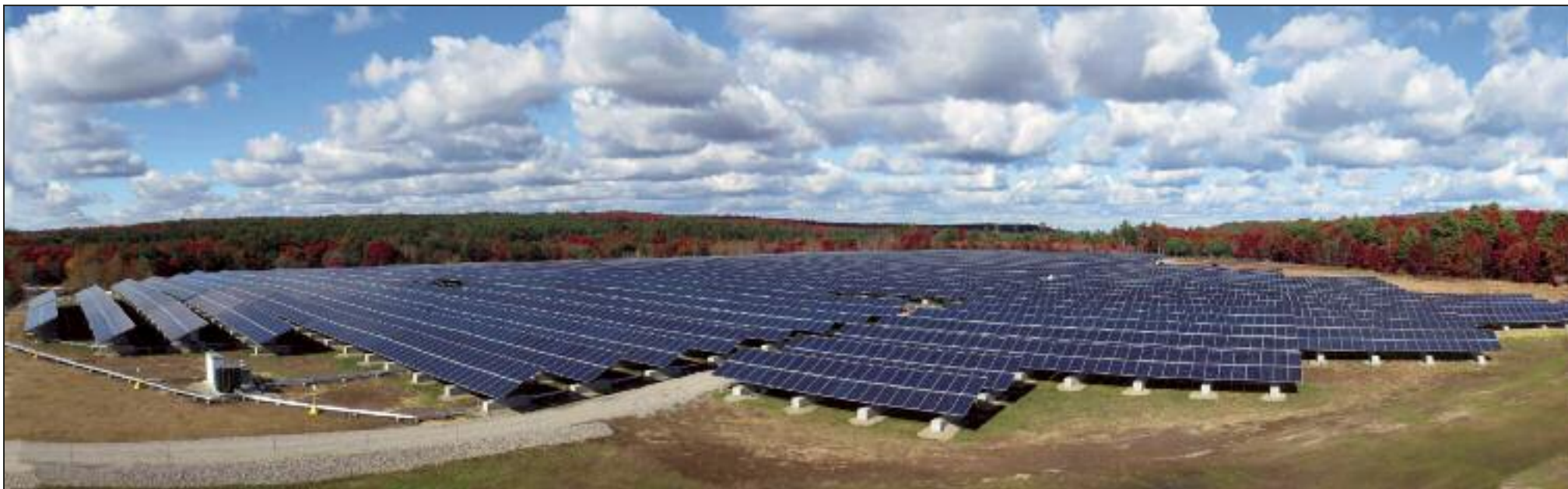
Washington Gas Energy Systems hired Sundurance Energy to construct this 4-megawatt solar array built on a Marshfield, Massachusetts capped landfill. The solar array consists of 13,518 panels covering 13 acres of land with Garden State Engineering, Surveying and Planning, Inc. providing the foundation design required to distribute the power produced by the solar panels at this site.
