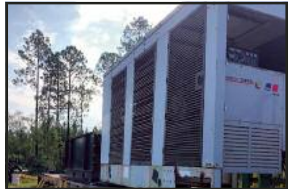
DETROIT DIESEL 425KW GENERATOR 240/480V three phase, 500 amps.
