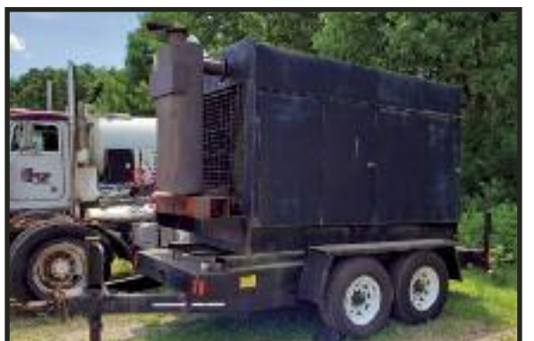
LEROY SOMER PORTABLE 250KW GENERATOR 60 Htz 3 phase 240/480 Volts John Deere Motor.
