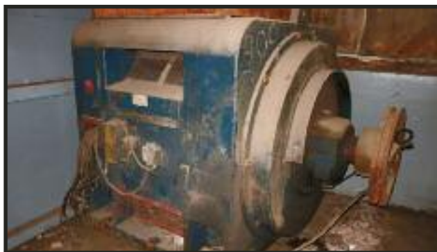
Fairbanks Morse 3,000HP Motor. 869 RPM. Stored indoors, but hasn't been turned.
