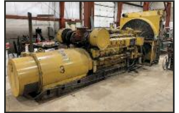
CAT DIESEL SYNCHRONOUS AC GENERATORS 1250KW. 2400/4160V. 3 available.
