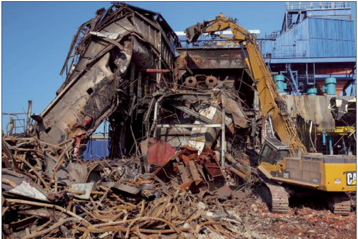
While regulations continue to be enacted, the C&D recycling industry could use more strategic regulation to improve diversion rates. PHOTO COURTESY OF ADAMO GROUP
