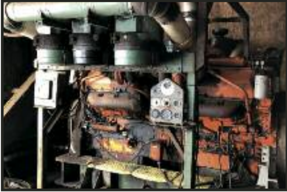
WAUKESHA 12 CYLINDER DIESEL ENGINE
