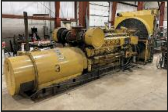
CAT DIESEL SYNCHRONOUS AC GENERATORS
