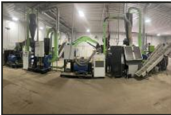
2017 STOKKERMILL COPPER RECOVERY SYSTEM
