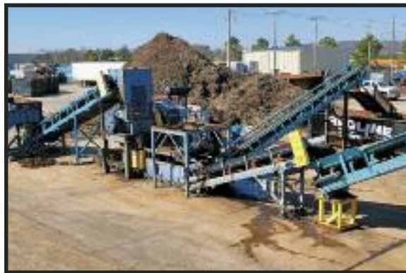
AMERICAN PULVERIZER 4800 RING MILL SHREDDER
