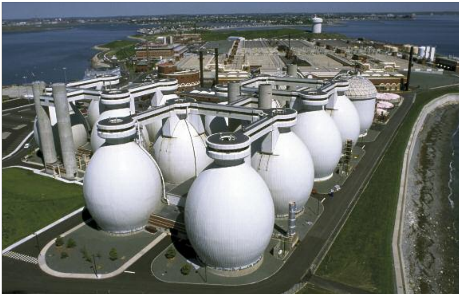
Egg-shaped digesters originated in Germany in 1950s and they are used to treat sewage works sludge as well as other organics that break down and produce biogas.
