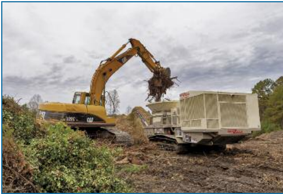
CW Mill Equipment Co., Inc.
