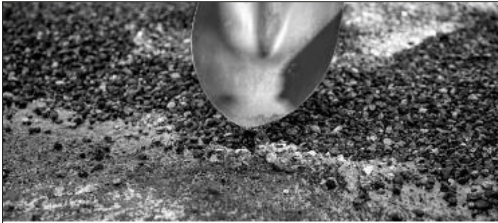
Installation of rubber modified chip seal on 7 Mile Road in Bay County, Michigan.
