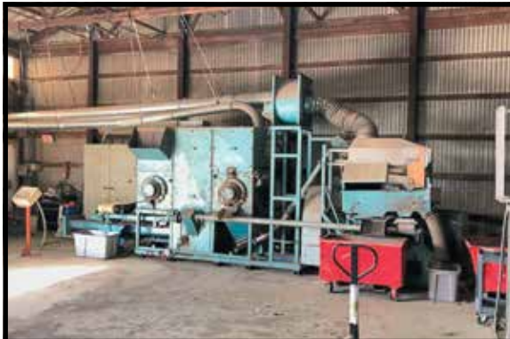
ELDAN 400C CABLE SEPARATION PLANT INCLUDES RASPER, GRANULATOR, AND MORE!
